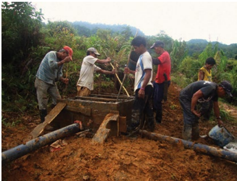
Men from Maling constructing one of the six distribution boxes of the irrigation system through angkas (Barangay Maling)
