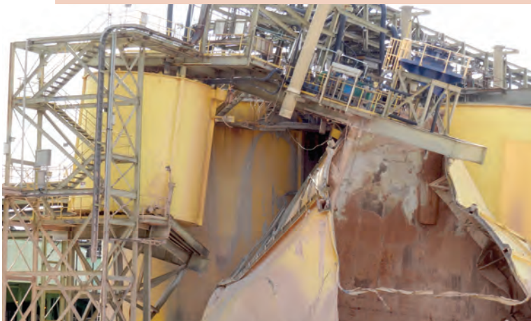
A massive uranium leach tank failed spilling highly acidic uranium slurry.
